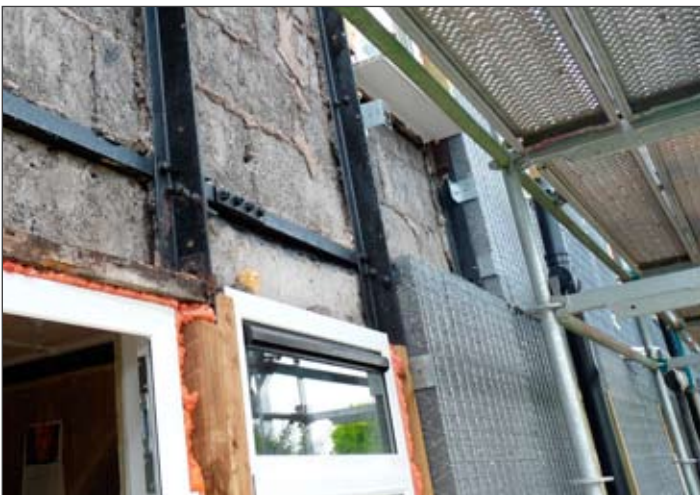
Shear receiver brackets and structural insulated cladding panels being installed between the steel columns of a stripped Dorlonco property.
